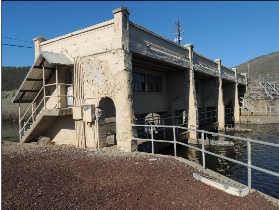
Figure 6: Pit 1 Gatehouse 9-10-11, April 2014. Note concrete spalling on exterior façade.
