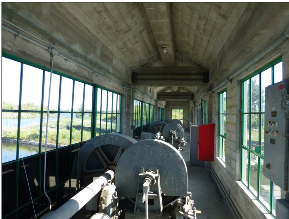
Figure 29: Interior of Gatehouse 1-2-3 showing equipment that black film applied to window panes hides from public view on the upstream side, May 18, 2016.
