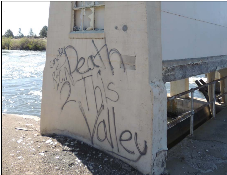
Figure 25: North side Gatehouse 1-2-3, April 2014. Note loss of texture already present on lower half of the exterior wall.
