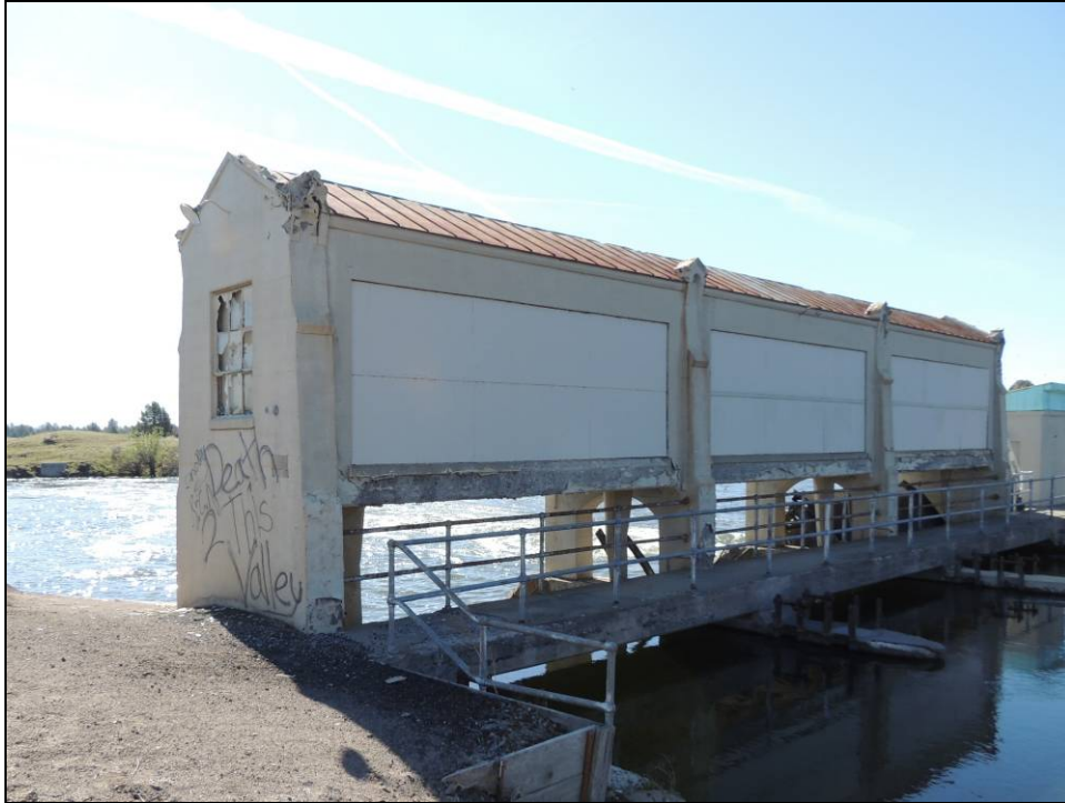
Figure 13: Pit 1 Gatehouse 1-2-3, April 2014. Note covered window bays, broken window panes, and heavily deteriorated window sills and ornamental pinnacles.
