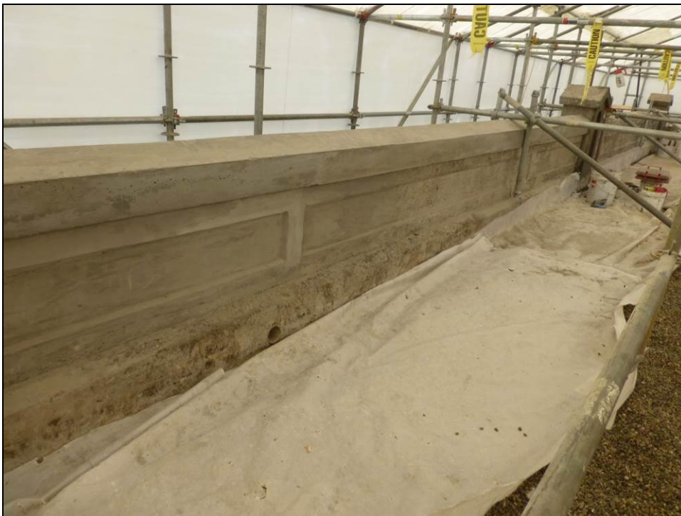
Figure 18: Section of upper level of Gatehouse 9-10-11 nearing completion of reconstruction (see Figure 16 ), May 19, 2016.
