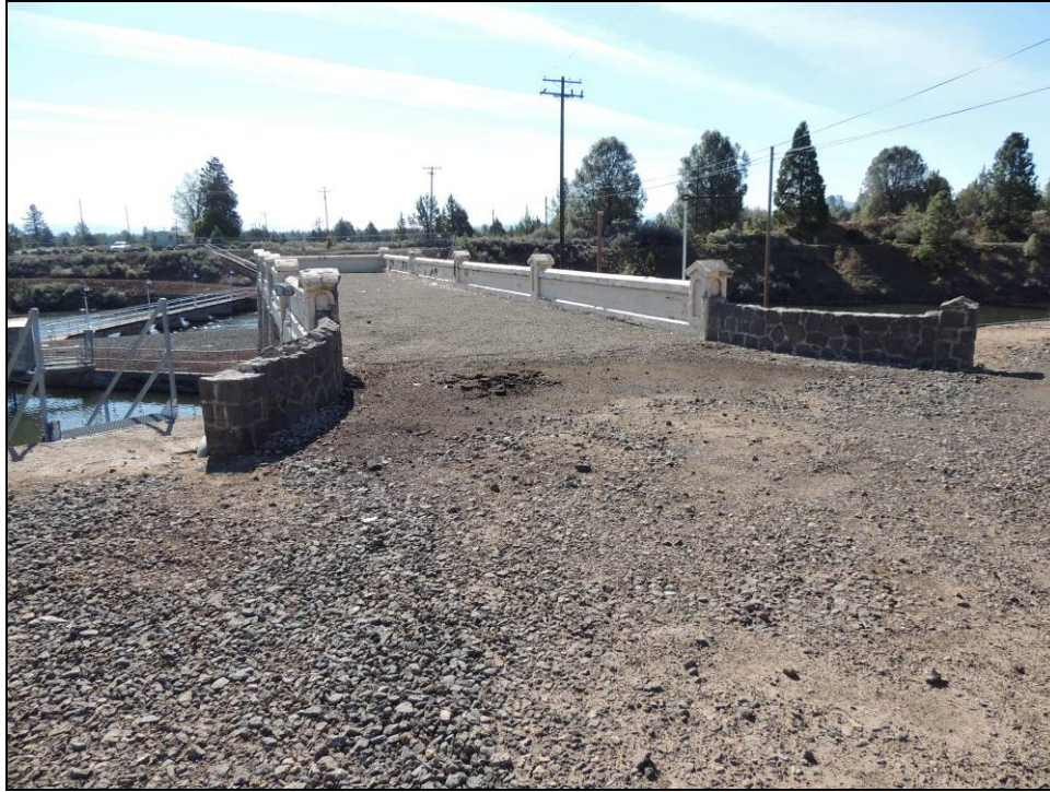
Figure 12: Remaining bridge approaches on west side of Pit 1 Gatehouse 9-10-11, April 2014. Note deteriorated ornamental end caps on stone approaches.
