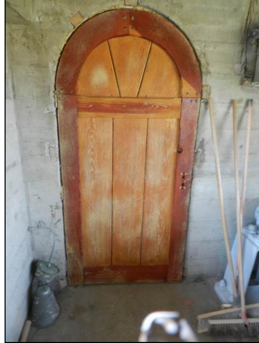
Figure 35: Original door on west side of Gatehouse 9-10-11, stripped and coated with a clear coat, August 16, 2016.
