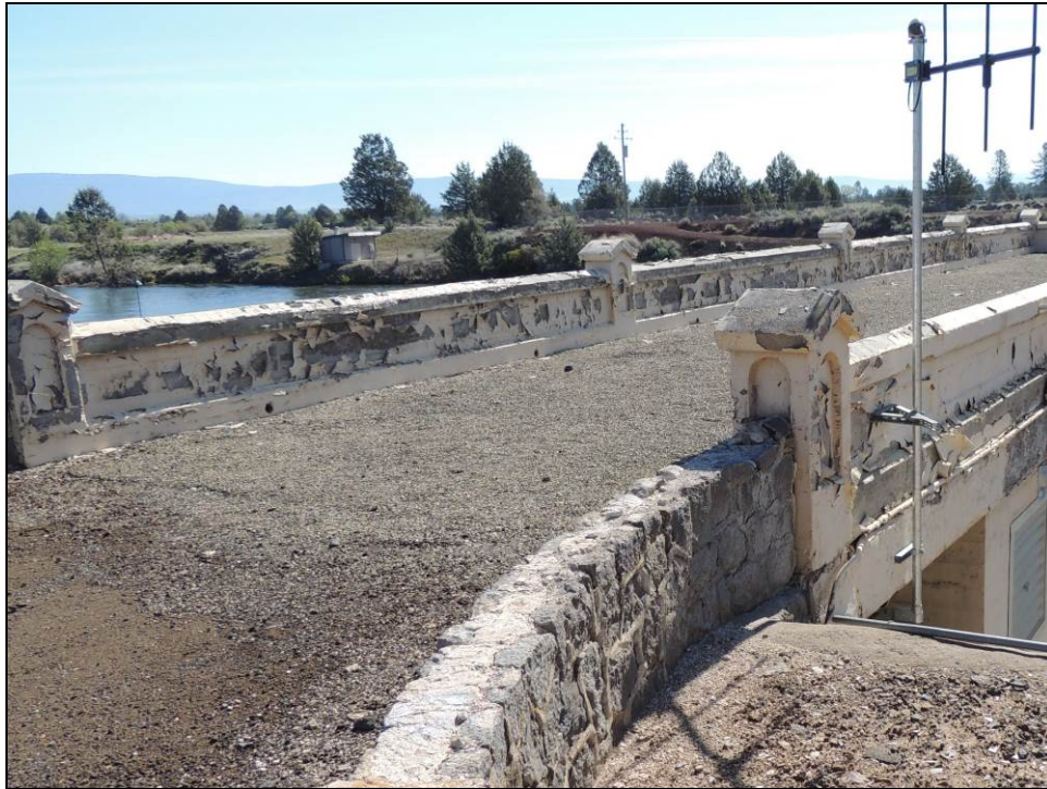
Figure 11: Pit 1 Gatehouse 9-10-11, April 2014. Note extensive degradation and peeling along interior retaining walls of former road deck.
