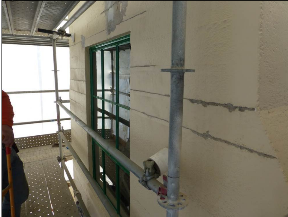
Figure 24: Trial area where AST has applied indentations to restore the horizontal appearance of board-form impressions in the concrete, January 27, 2016.
