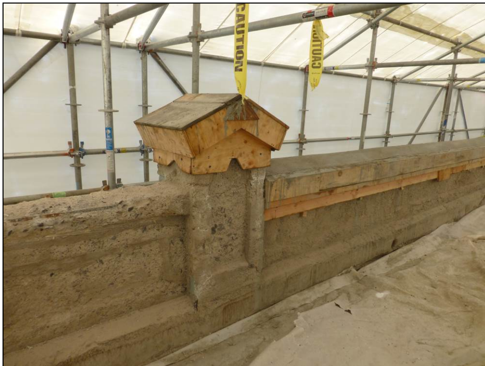
Figure 22: Wood form used to reconstruct ornamental pinnacles and railing details at Gatehouse 9-10-11, May 18, 2016.
