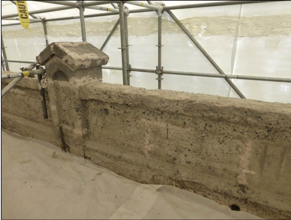
Figure 17: Section of upper level of Gatehouse 9-10-11 that has been subject to dental removal of degraded concrete, May 19, 2016.
