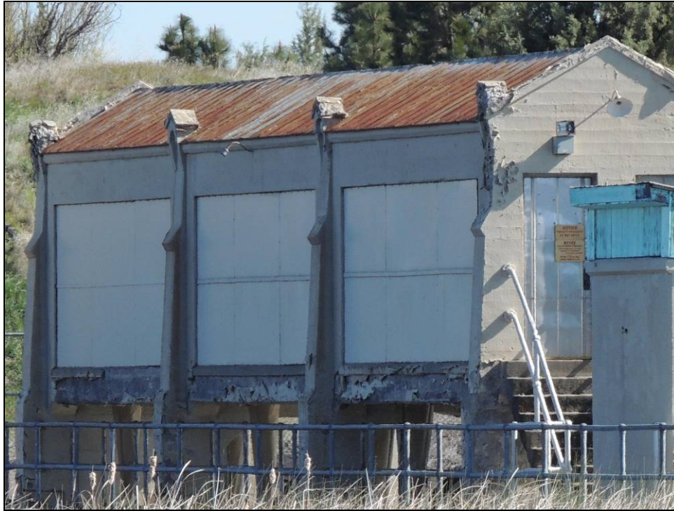
Figure 15: Pit 1 Gatehouse 1-2-3, April 2014. Note significant spalling of ornamental concrete pinnacles at roofline, and at and below sills, covered windows and deteriorating tin roof.
