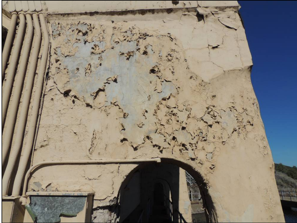
Figure 8: Detail view of concrete spalling on northeast corner of Pit 1 Gatehouse 9-10-11, April 2014.
