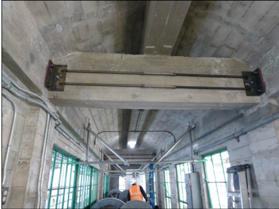
Figure 27: Reinforcing bars installed at interior of Gatehouse 1-2-3 do not penetrate the building to the exterior, January 27, 2016.
