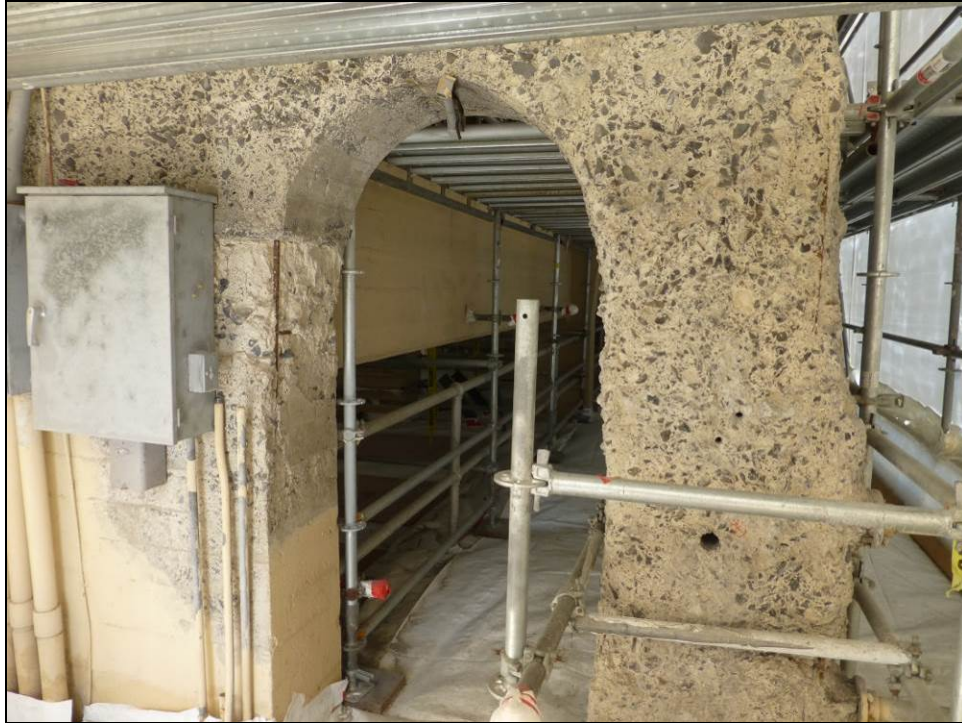
Figure 19: Heavily degraded column on east end of upstream side of Gatehouse 9-10-11 after dental removal of deteriorated concrete, May 19, 2016.
