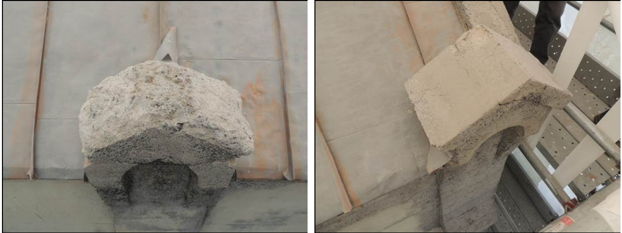
Figure 21: Ornamental pinnacle at Gatehouse 1-2-3 after deteriorated concrete removed at left; intact pinnacle at Gatehouse 1-2-3 used for mold at right.
